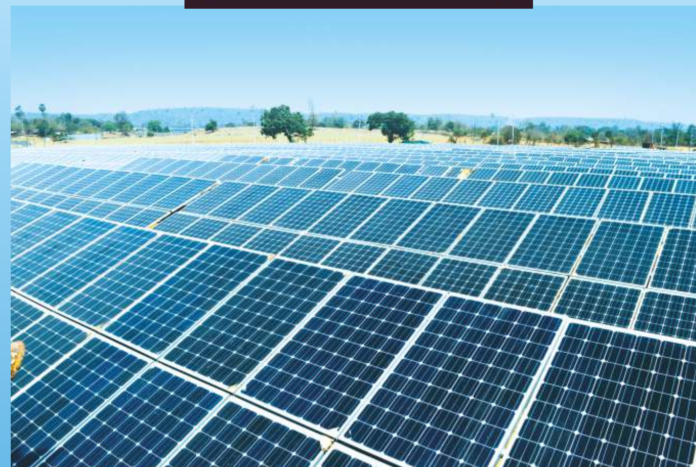
Solar Panel, Dadra & Nagar Haveli
